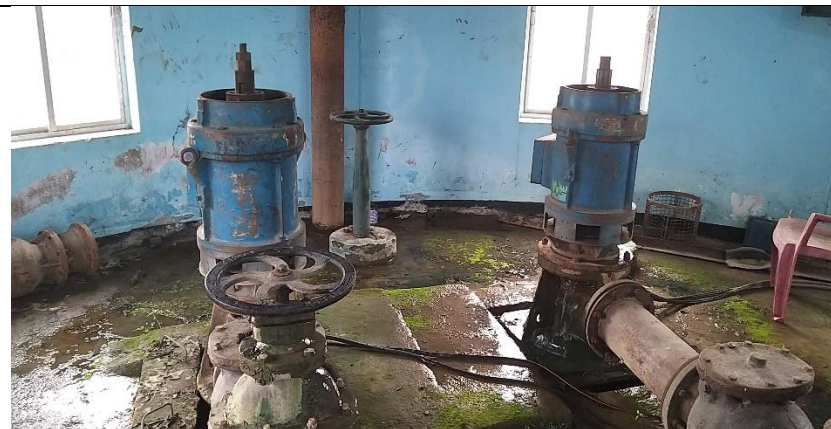
Intake Raw water pump
