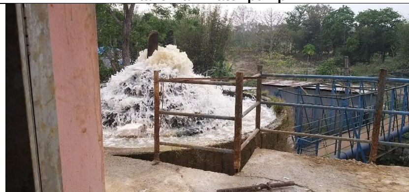
Cascade Aerator – WTP
